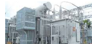
①変圧器外観
