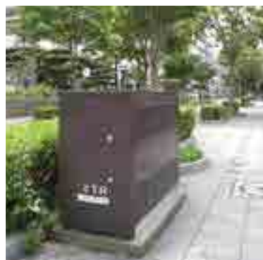
変圧器塔 Pad-mounted transformer
